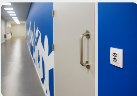
RFID antennas and readers are seamlessly integrated into walls and ceilings.
